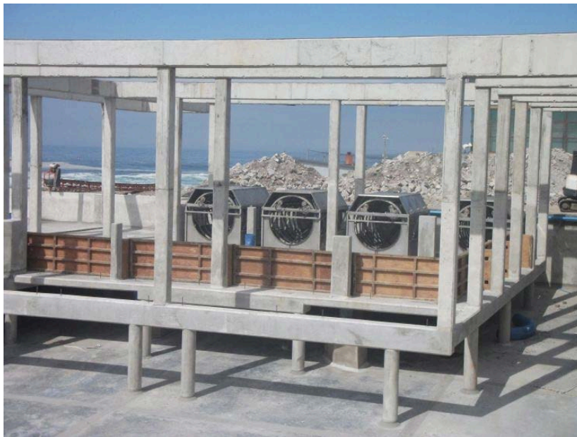
The new drum filters, for further cleaning of water.
